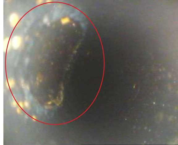
Figure 4: APR Tube #112, 44% wall loss (pitting) at 7.56m
