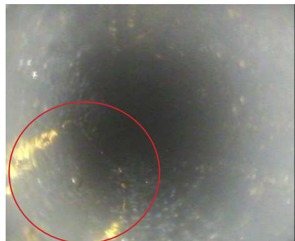
Figure 6: APR Tube #126, 29.4% wall loss (pitting) at 6m
